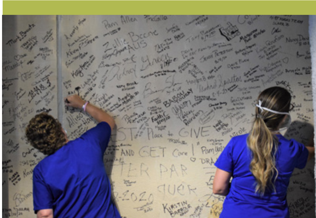
Hospital staff members sign a wall in a new lobby area under construction at Duke Raleigh Hospital.
